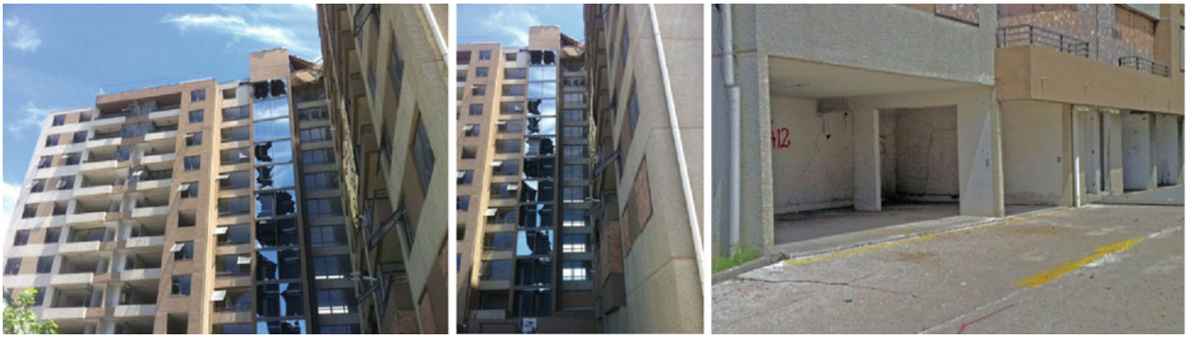
Fig. 14.4 Damage observed in 12-storey reinforced concrete building
